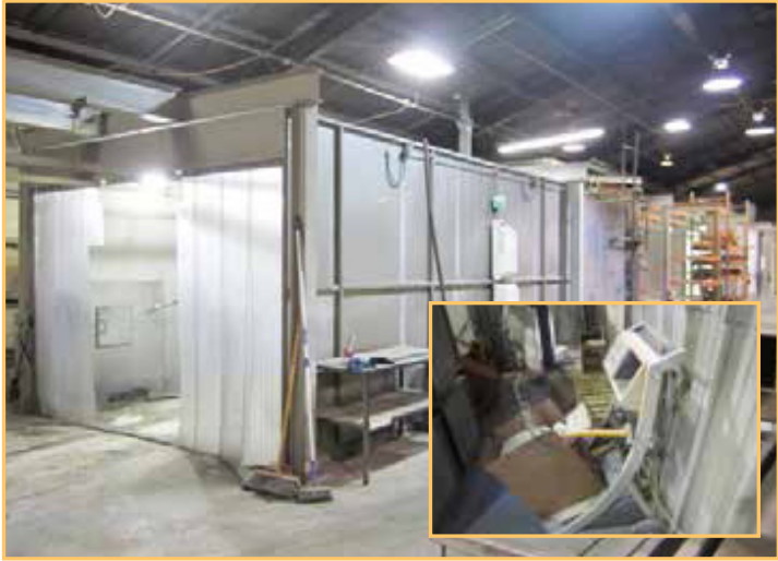
COL-MET POWDER COAT SPRAY BOOTH W/(3) ITW PAINT SPRAYERS
