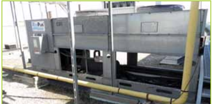
(29) KRACK, LARKIN, REF PLUS, AND KEEP RITE 2, 3, 4, 5, AND 6-FAN FREON COOLER AND FREEZER BLOWERS WITH COMPRESSORS AND EVAPORATORS.
