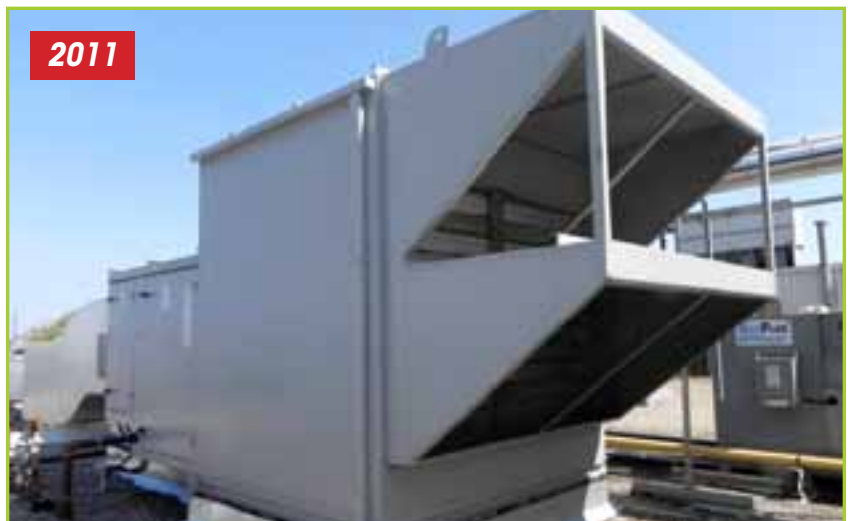
2011 ENGA NATURAL GAS AIR HANDLER
