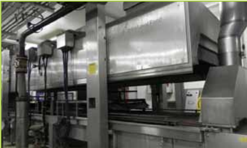
TETRA LAVAL / KOPPENS STEAM & ELECTRIC HLT S/S OVEN
