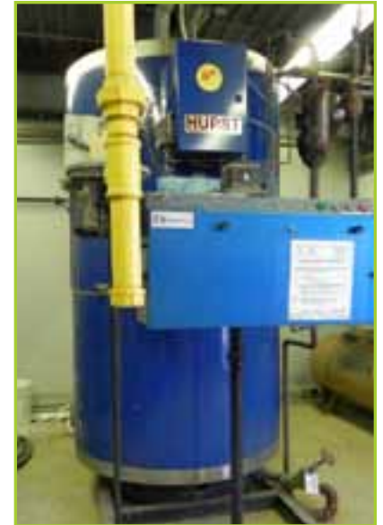
HURST 50 HP BOILER
